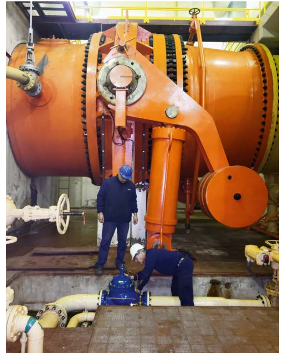
The Water & Sewage Division was instrumental in protecting the Futaleufú hydroelectric power plant's critical components against cavitation effects
