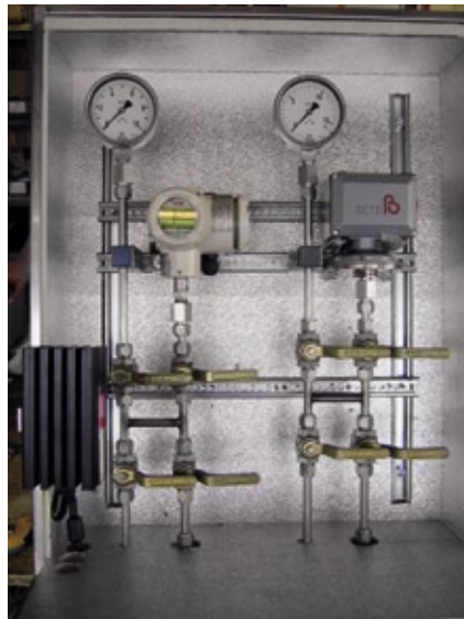
A pressure transducer, which converts the physical input signal to an analogue signal (4-20 mA), is located in the left corner. The device installed on the right side is a pressure switch that converts the physical input signal into a binary signal (0 or 24 VDC).
